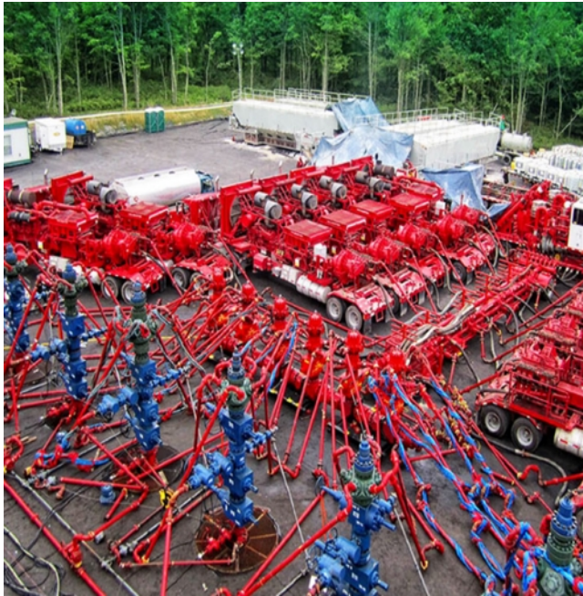
Figure 3: A Typical Frac / Pressure Pumping Setup
